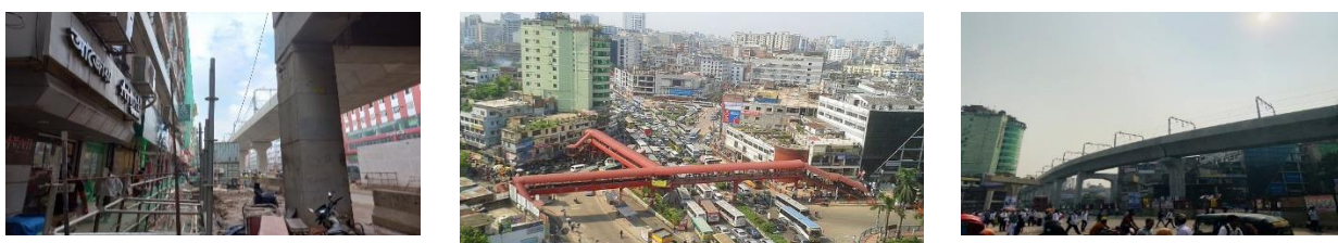
Figure 17: Blocked and Narrowed Footpath for Pedestrian Movement Impact of COVID-19 in MRT Line-6 Construction
